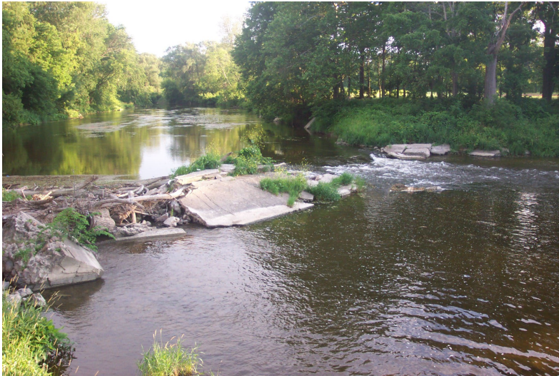
Parshallburg’s failed but not entirely dismantled “Dam”
