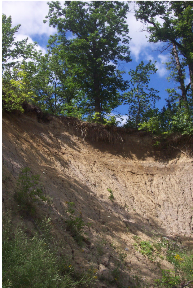
Erosion Scar north of 6 Mile Creek Bridge
